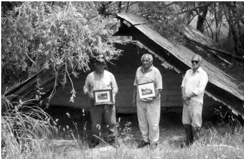
Photo: Three members of Te Aitanga-a-Mahaki outside the abandoned meeting house at Mangatu which was all but destroyed by valley infilling and flooding.
