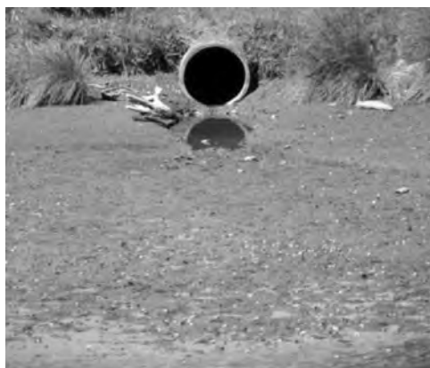
Figure 10.2 – Stormwater or wastewater?
