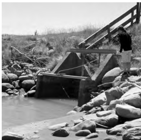
Figure 4.5 – The floodgate and stopbank across the Awapuni Creek
